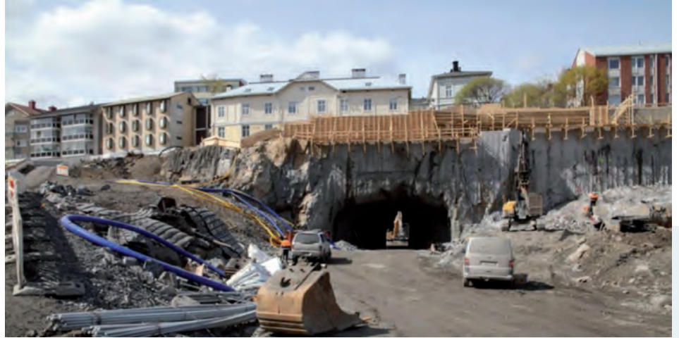
Figure 10 : A traffic tunnel heading in Finland. Photo courtesy of City of Tampere. Excavation work done by Lemminkäinen Oy
