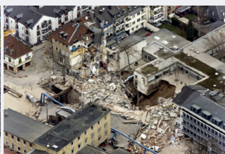
Devastating collapse of an open cut crossover and sump structure in Cologne in 2009
