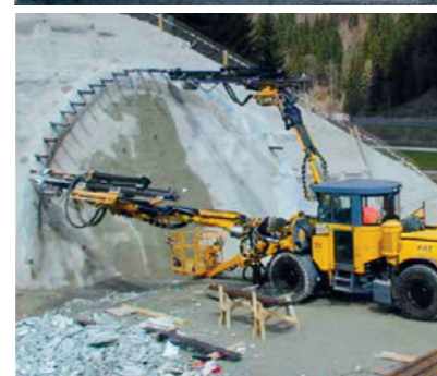
From top: Studying in the art of NATM excavation; All aspects of NATM excavation are covered
