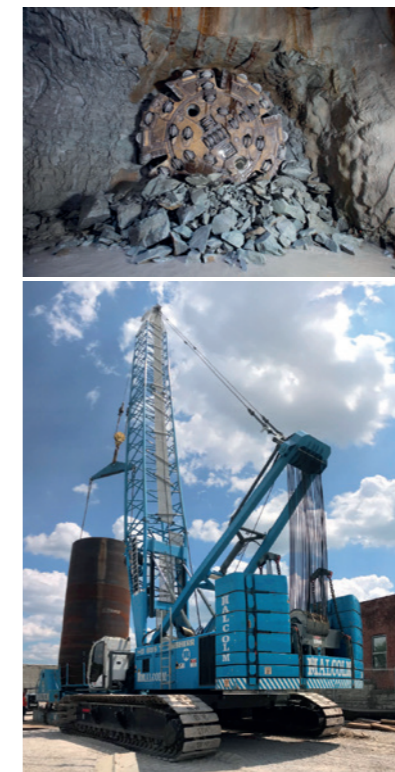
From top: Breakthrough on White River section; Crane-mounted oscillator installs drop shaft cans
