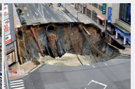
Many a sinkhole has provided a hard lesson for competent excavation
