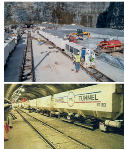
From top: Mining Equipment loco and muck cars in action; Mühlgäuser operations on the Channel Tunnel
