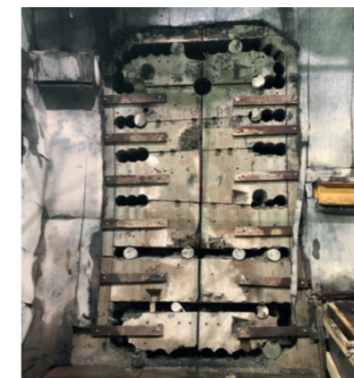
From top: Frozen cross passage face; Extra support frame; Breakout of segmental lining
