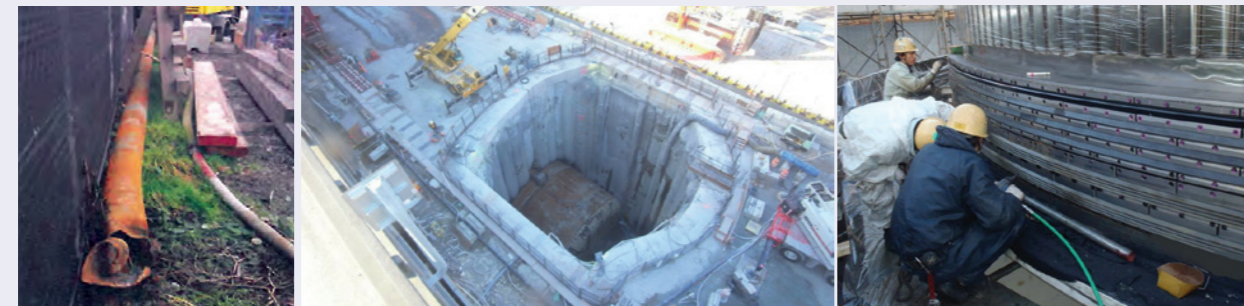
Top from left: Alleged culprit of the TBM damage and breakdown; Claims were to cover costs of the recovery shaft and repair of the stricken TBM; Repair included fitting a replacement main bearing; Below: Replacement highway route under the streets of downtown Seattle; Seattle waterfront before and after the elevated highway viaduct demolition
