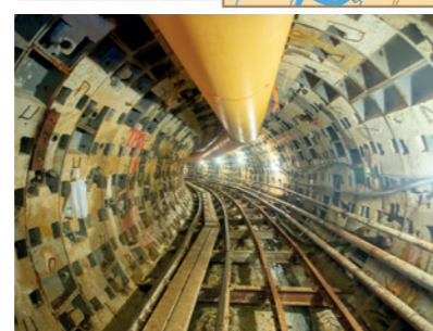
Fig 1. Tight curve TBM drives follow public road easements; Short steel segment rings follow the TBMs through the sharp radius curves
